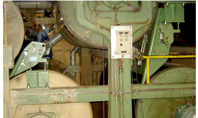
EVsf web stabilizers were installed to support sheet run at single felted drying section
